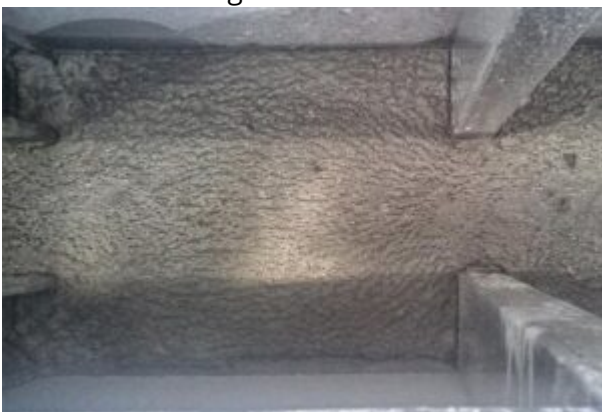
Light weight concrete applied to the inside of a Double Wall structure.
